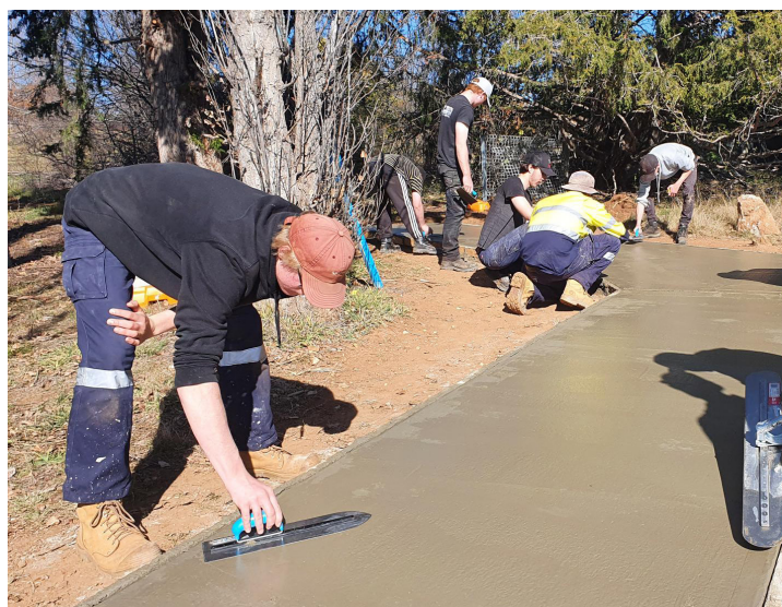
Construction students working on a new path at the back entrance of the school
